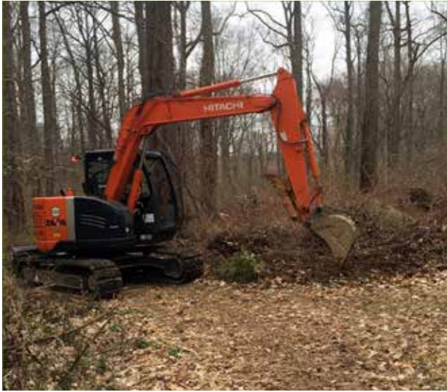
Figure 2. Heavy equipment used by the landscape contractor to clear the site to bare ground. [Photo by C. Johnston, 4/14/15.]
